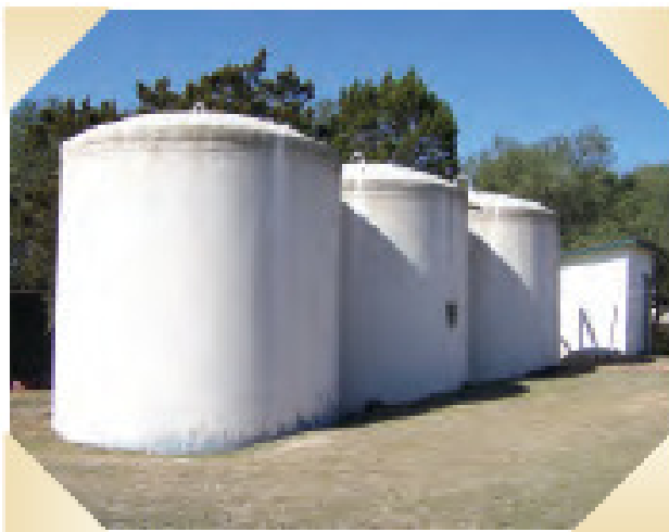
Rainwater collection tanks.
